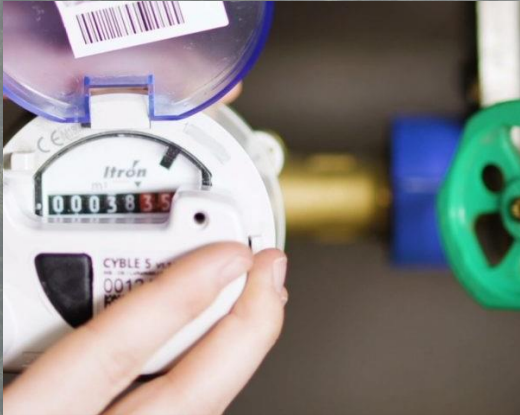
Saving resources with smart water meters
